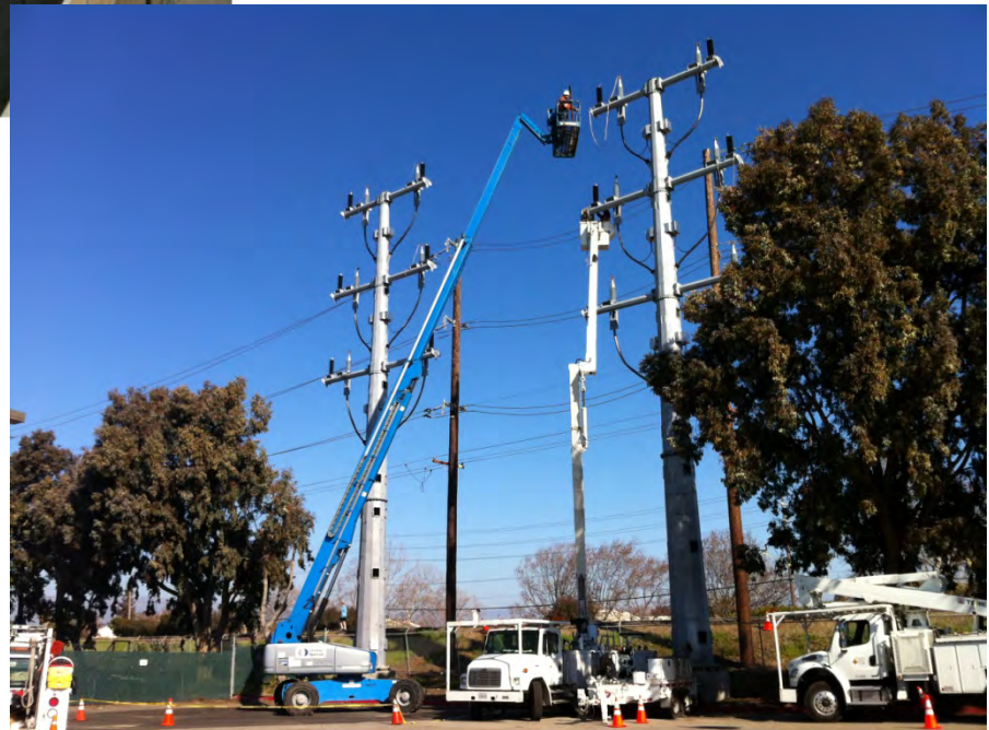
60kV Riser Poles
